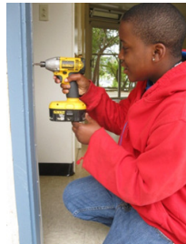
SYEP Participant Steven Louis helps weatherize doors for the Marin Housing Authority Greenovation Project.
